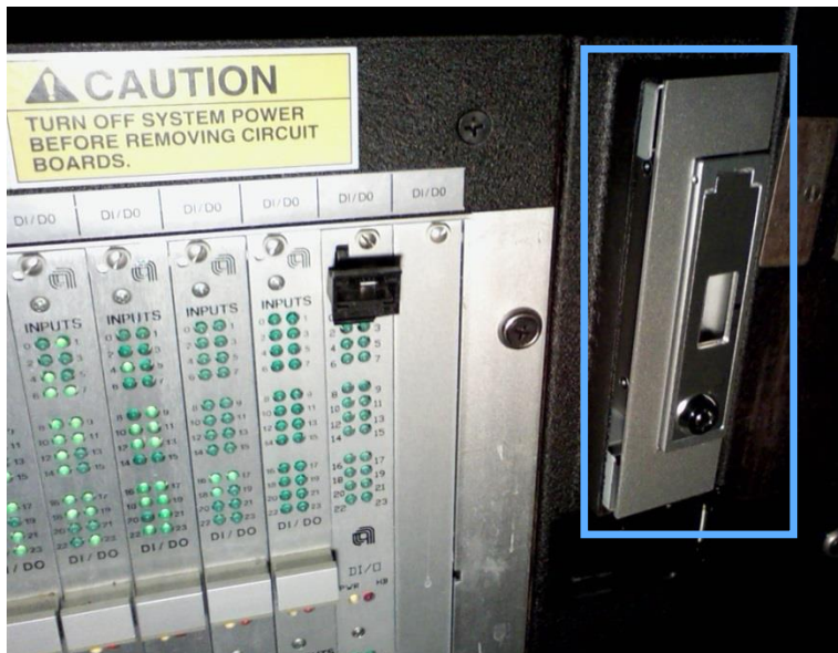
Ref. Installed in CVD equipment
